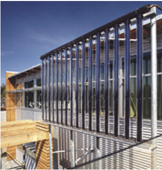
An active solar hot water system serves as a source of heat for the building.
