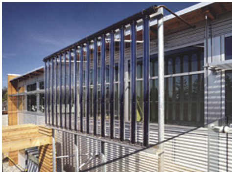
Figure 6: An active solar hot water system at the City of White Rock's Green Operations Building serves as the primary source of heat for the building.
